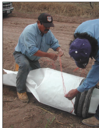
Figure 5b. Using a corrugated PVC pipe to connect two rolls of poly-pipe.
